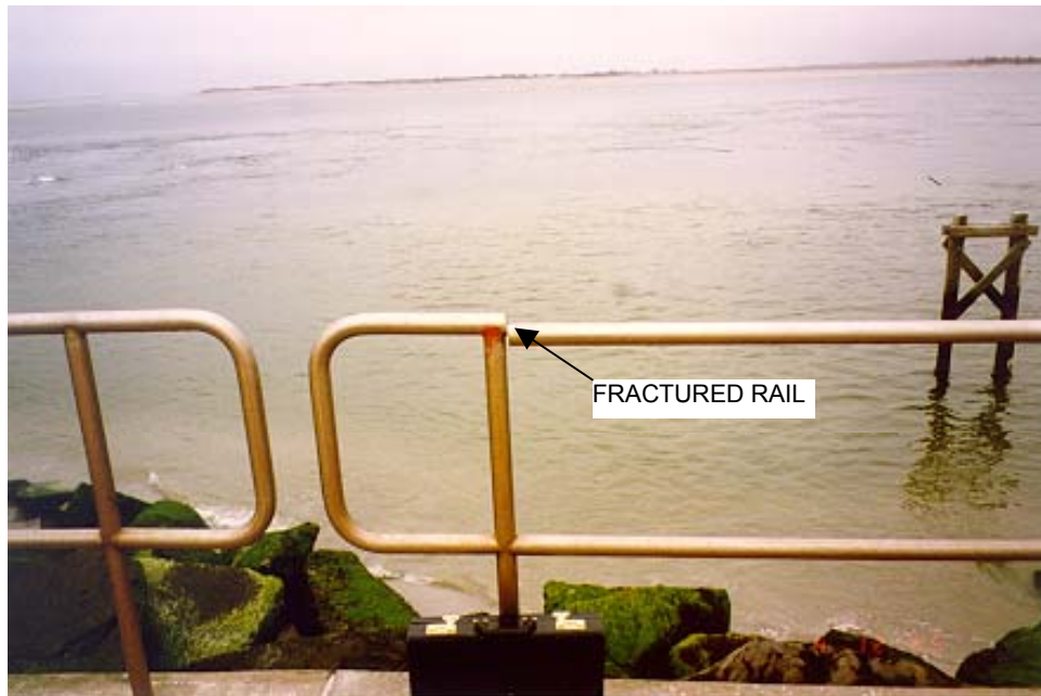
Figure 8-16. Cracked steel handrail
