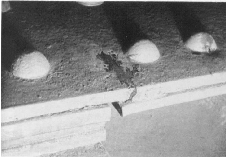
Figure 3-2. Fatigue crack at tack weld on a riveted member
